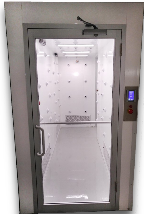
Air Shower Tunnel Entrance
